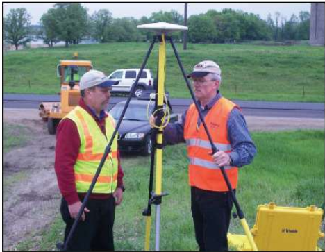
Figure 13. A Trimble GPS base station (ICPF MnDOT demo).
