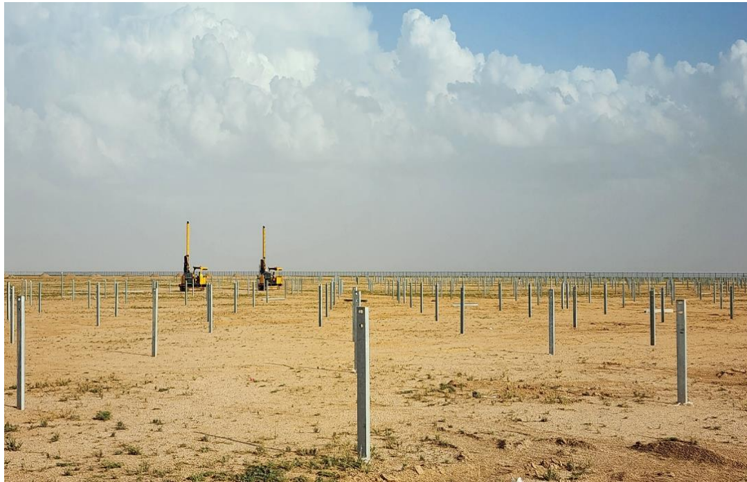
PV Modules Mounting Structure Posts
