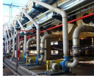
Oil Pump Station & Gas Pressure Boosting Stations
