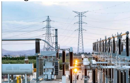
Power Plants, Power Transmission Lines and Substations
