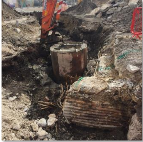
Kirtling Street Obstructions
