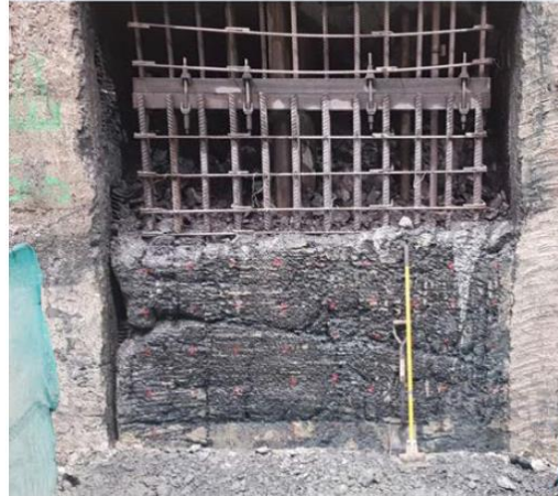
Chambers Wharf Diaphragm Wall Collapse
