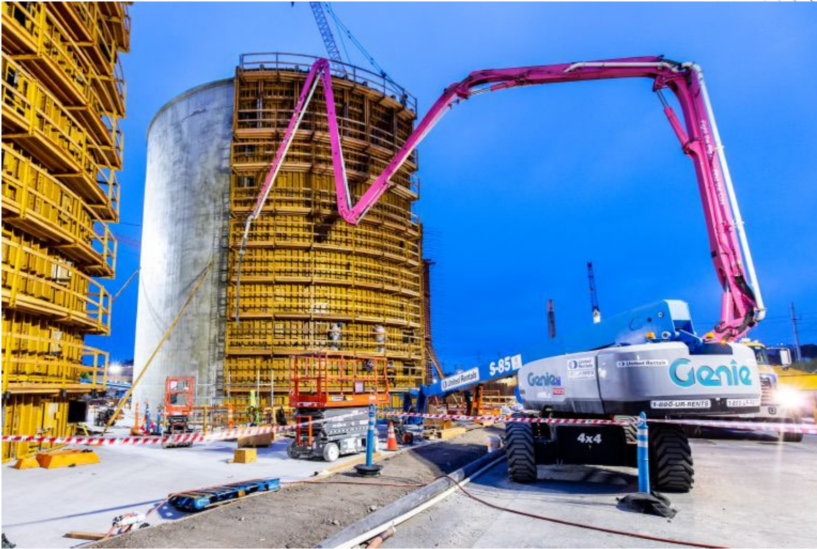
Digester Tank No. 4 core wall pour in the early morning hours of July 19th, 2023.
